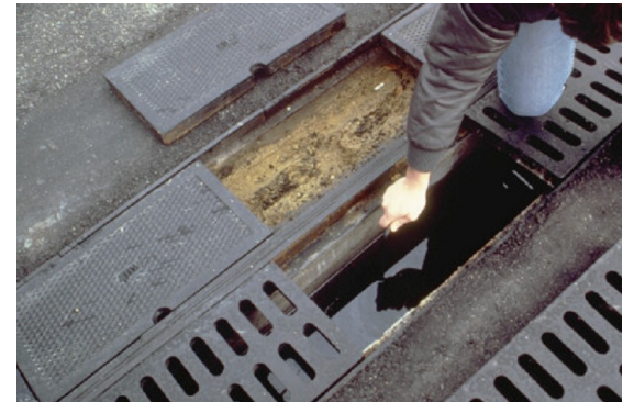
Perimeter Sand Filter
